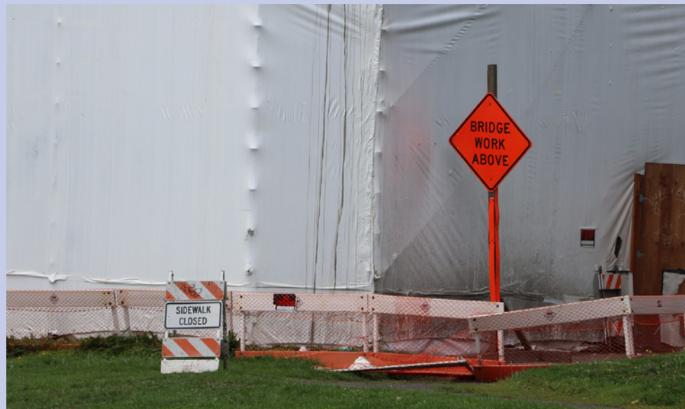
A photo of the St. John’s bridge under routine bridge repair courtesy of ODOT’s Fix-It Bridge program. Photo courtesy of the Oregon Department of Transportation.
